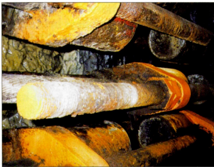
Fig. 11: Adjustable connection at the anchorages installed in the early 1980s
