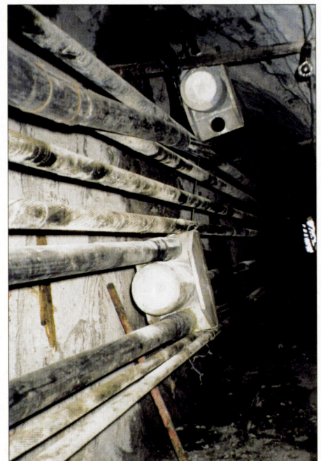
Fig. 13: New anchoring system with prestressing cables (the tunnel entrance can be seen on the right)
